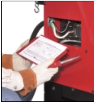
Easily accessible voltage reconnect panel.
